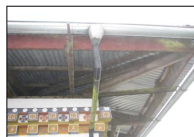
Rain water harvesting at Yongla
