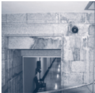
Centre Block—Water infiltration has caused rust from structural steel to permanently stain stone interior finishes in some areas, including chambers and ceremonial spaces.
