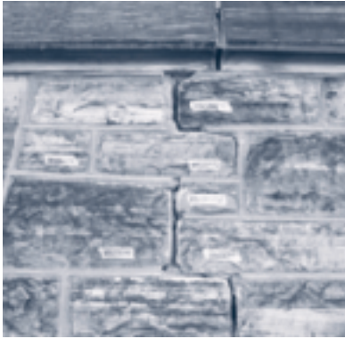
West Block—Water infiltration into main structures is eroding mortar.
