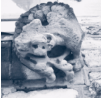
West Block—Permanently damaged carved elements of the historic structure need to be rebuilt.
