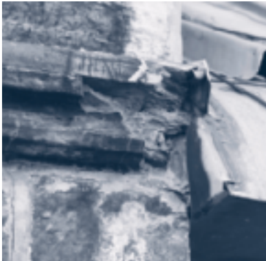
Centre Block—Permanently damaged sandstone cornices and carved elements of the historic structure need to be rebuilt.
