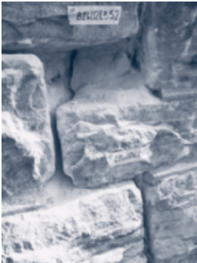
West Block—Water infiltration into main structures is eroding mortar.
