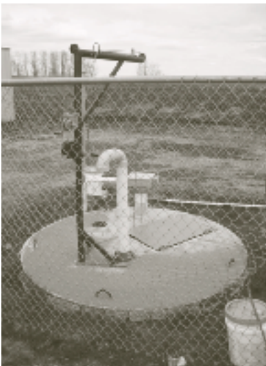
Protected water facility at a Correctional Service Canada institution
