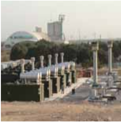
A landfill gas generating station.
