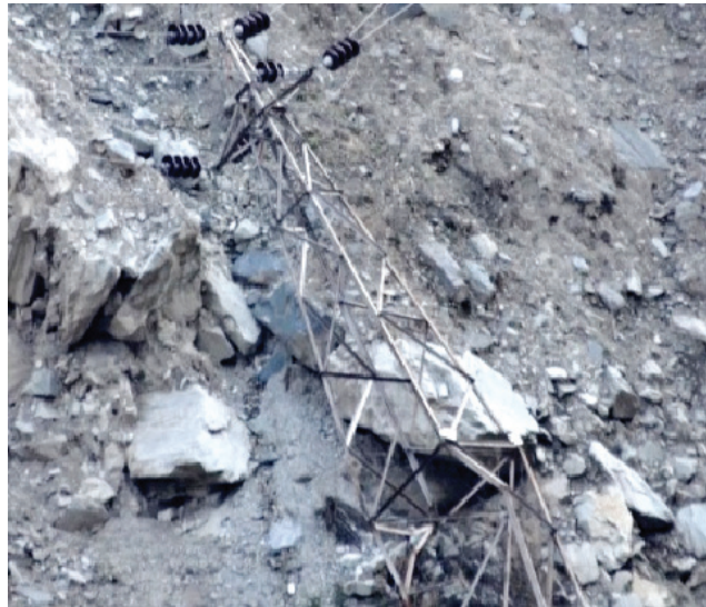
Unrestored electricity transmission line at Khet (Pithoragarh) 03.01.2015
